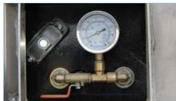
Air gauge and dump valve.
